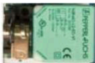
Escalator Missing Switch
