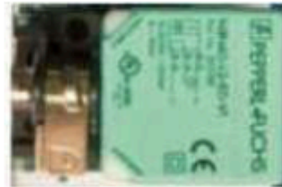
Escalator Missing Switch
